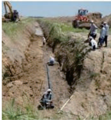
Construction of subsurface drainage (New construction project with financial assistance from aid agency)
