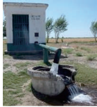
Existing vertical drainage (Power costs are high and operating hours are limited)
